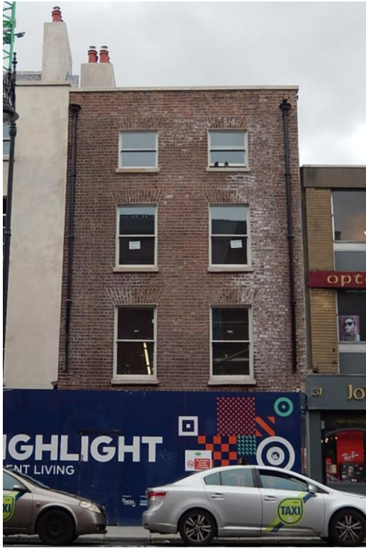
View of newly repointed facade with reinstated wigged joint and new sash windows
