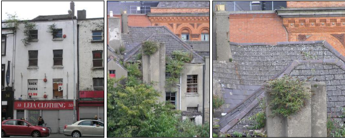
Photos of 33 Thomas Street taken from 2012 Dublin Civic Trust Study showing early roof form.
